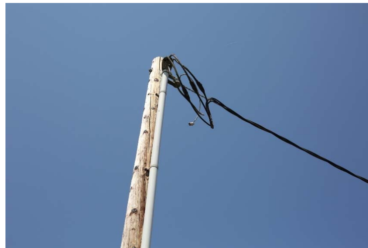
Broken Neutral Service Before Repair
